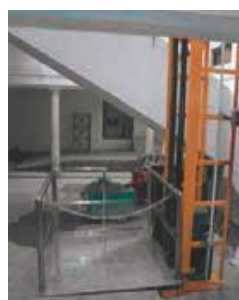
Single Mast Lift inside Building
